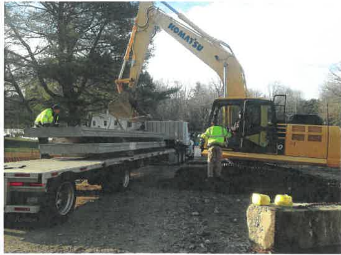
Figure 10 The bridge abutments were finished and the prefabricated decking was installed using a Town excavator which reduced the cost to the contractor, Contech.
