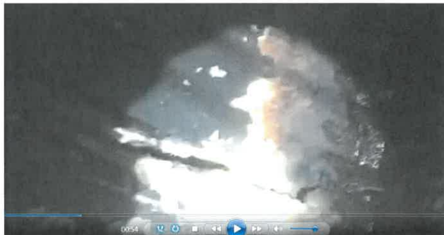
Figure 5 Picture of rusted out areas of the pipe under Cobb Road. There are numerous. The video is available on YouTube at https://youtu.be/Xs9bldTbMPE (the picture should be rotated... up is the direction of water flow).
