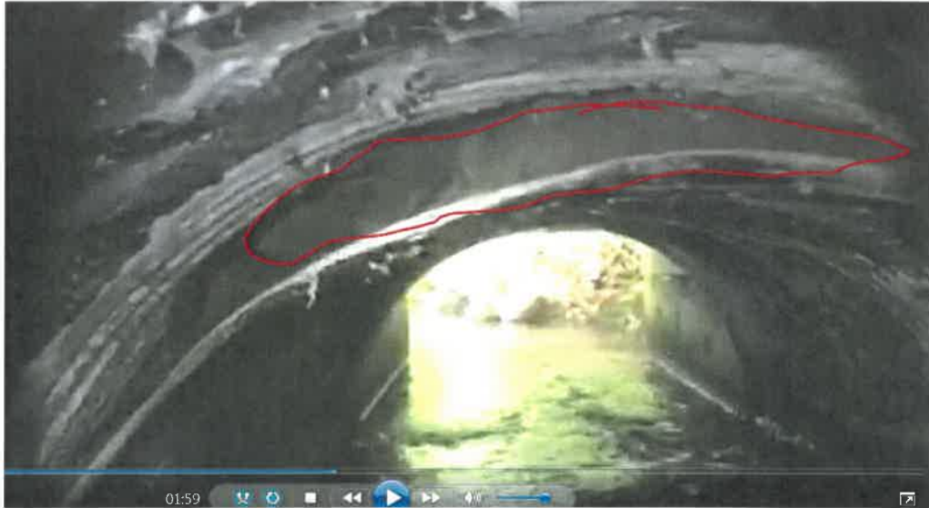
Figure 6 The outlet does not fit the pipe properly causing far more turbulent flow and reducing the pipes discharge/flow capacity. The video is available on YouTube at https://youtu.be/Xs9bldTbMPE .
